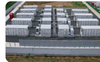
Wuhe Green Energy base: PV+ES Project
