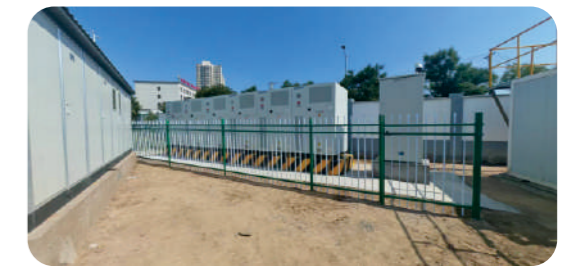
Shenmu Sewage Treatment Plant: Northern Shaanxi's First User Side Benchmark ES Project
