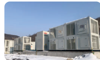
Shaanxi's first high power LFP battery + flywheel combined FM project
