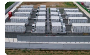
Wuhe Green Energy base: PV+ES Project
