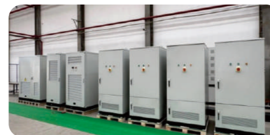
Taiwan Zero-Carbon Industrial Park: Region's First on/off grid switching ES Project
